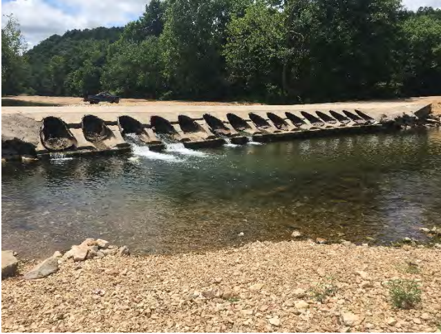
Figure 1: Example of a multi-culvert road crossing that likely blocks fish movement during most flow conditions. At the flow level in the image, all culverts have a vertical outlet drop and flow depths within the culverts are likely too shallow to allow fish movement.
