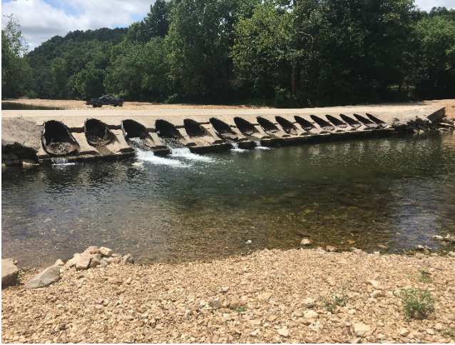
Figure 1: Example of a multi-culvert road crossing that likely blocks fish movement during most flow conditions. At the flow level in the image, all culverts have a vertical outlet drop and flow depths within the culverts are likely too shallow to allow fish movement.
